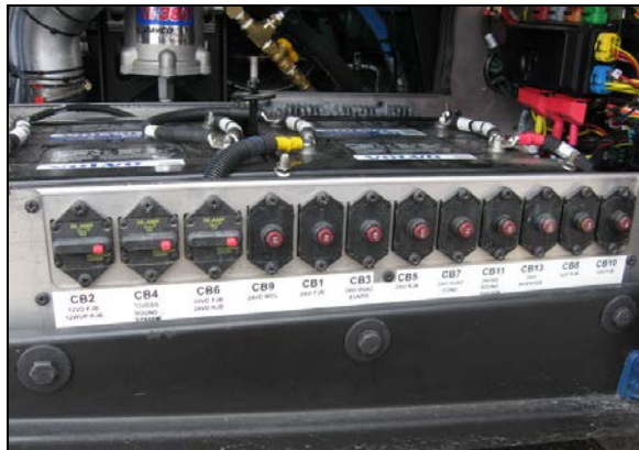
FIGURE 11: REAR ELECTRICAL JUNCTION PANEL
