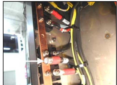
Figure 9: Power cable on main circuit breakers' bus bar.
