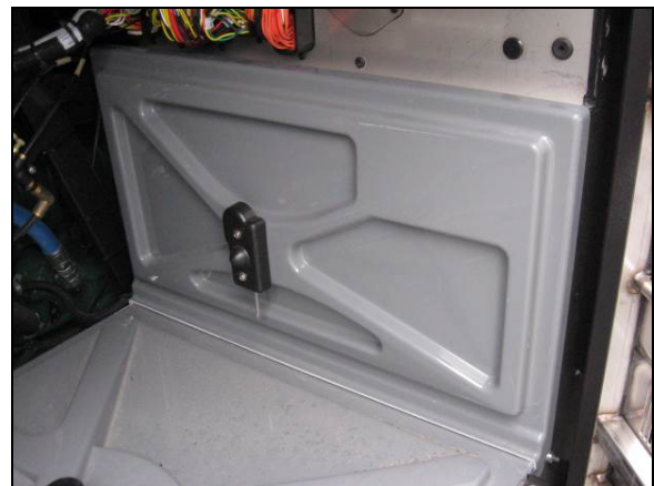
FIGURE 9: REAR ELECTRICAL PANEL
