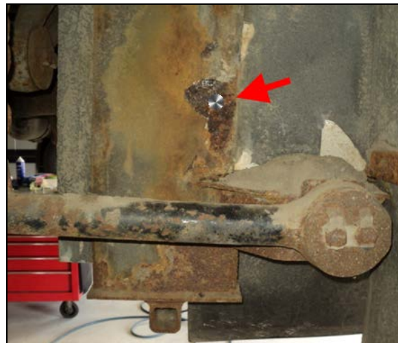
FIGURE 6: CLEANED SPOT ON STRUCTURAL MEMBER
