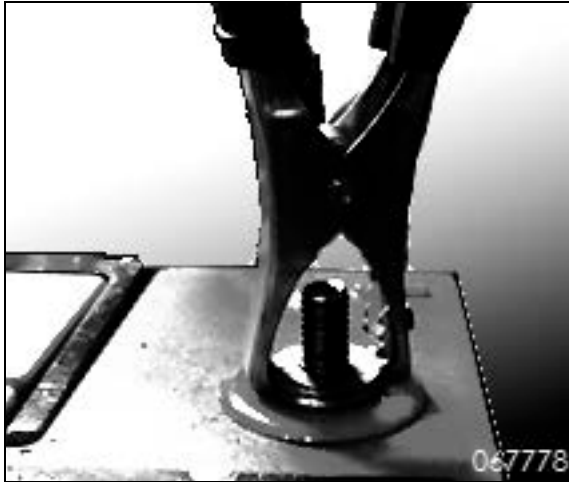
FIGURE 55 ALLIGATOR CLAMP POSITION- TYPICAL AGM BATTERY
