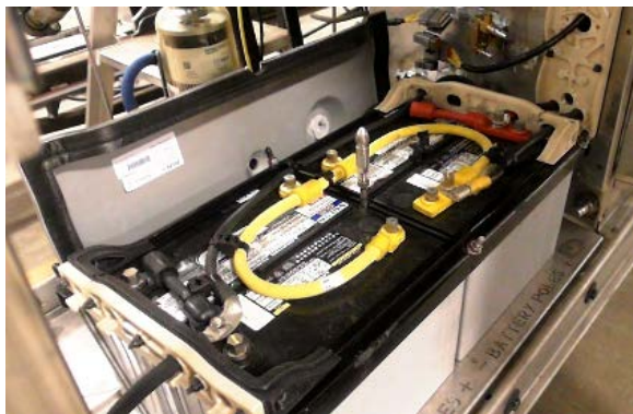
FIGURE 41: BATTERY BANK COVER REMOVED
