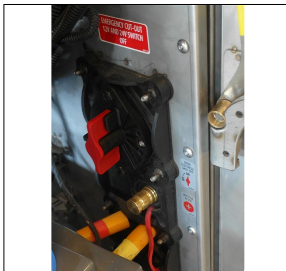
BATTERY MASTER SWITCH
