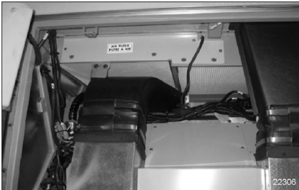
CABIN AREA AIR FILTER REMOVAL
