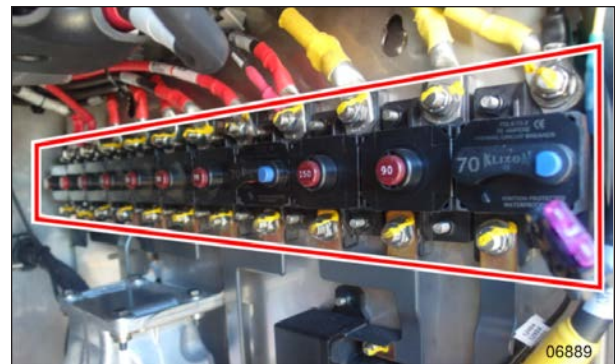
MAIN CIRCUIT BREAKERS IN MPC (TYPICAL)
