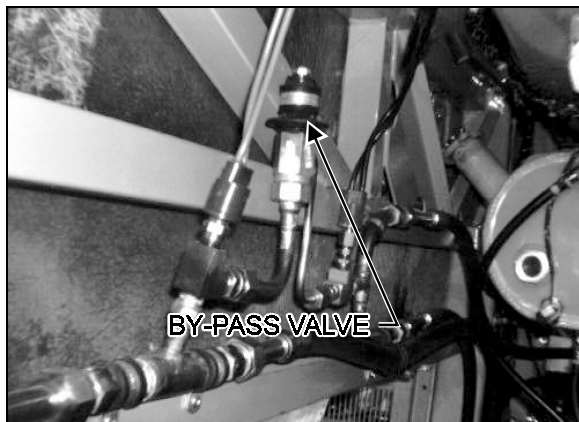
FIGURE 27: BY-PASS VALVE LOCATION 22078
