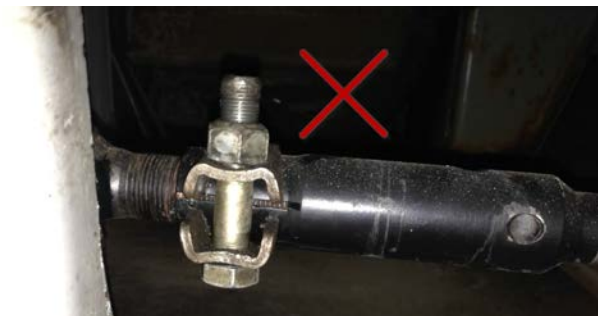
Clamp is bent. Replace clamp.
