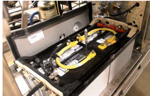
FIGURE 30: BATTERY BANK COVER REMOVED
