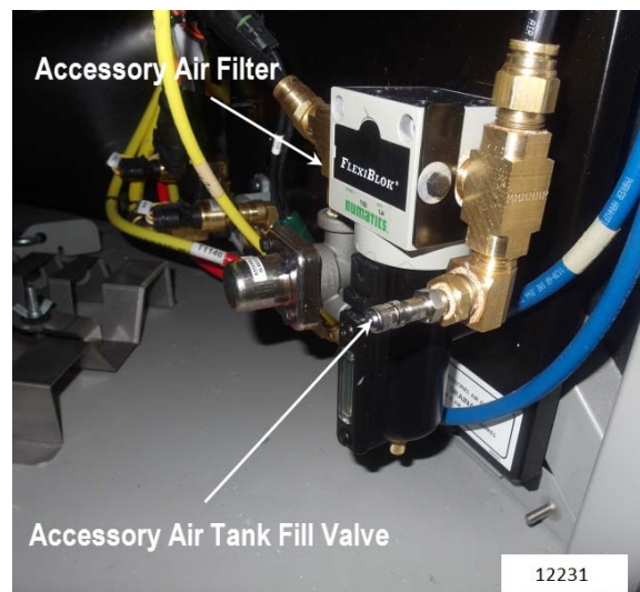
FIGURE 3: FRONT SERVICE COMPARTMENT
