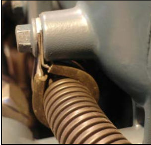
Figure 19: P-clamp with appropriate diameter prevents the power cable or corrugated protective sheath from moving and rubbing inside the clamp.
