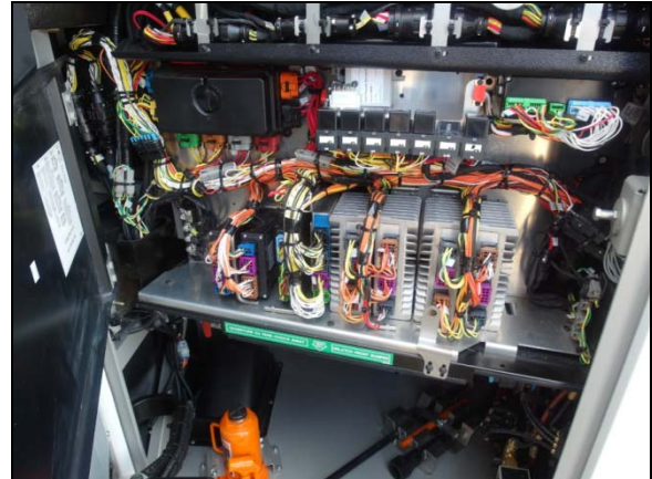
FIGURE 20: FRONT ELECTRICAL & SERVICE COMPARTMENT
