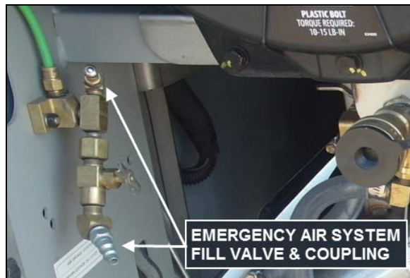
EMERGENCY AIR SYSTEM FILL VALVE AND COUPLING
