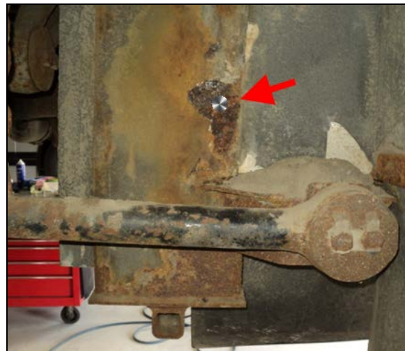
FIGURE 6: CLEANED SPOT ON STRUCTURAL MEMBER
