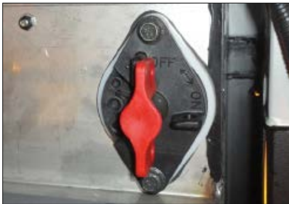
BATTERY MASTER SWITCH
