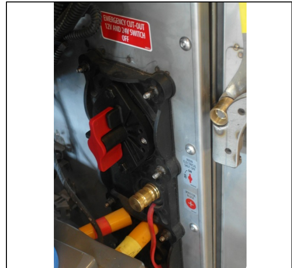
BATTERY MASTER SWITCH
