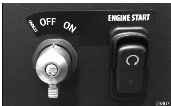
FIGURE 60: SWITCH ARRANGEMENT WITH STARTING MODULE
