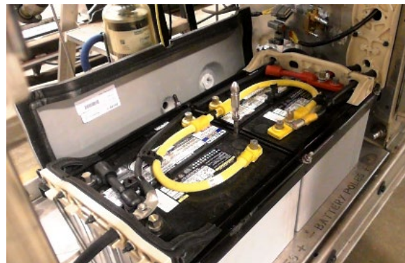
FIGURE 42: BATTERY BANK COVER REMOVED
