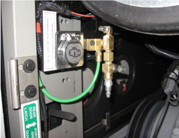
FIGURE 23 : ENGINE COMPARTMENT EMERGENCY AIR-FILL VALVE
