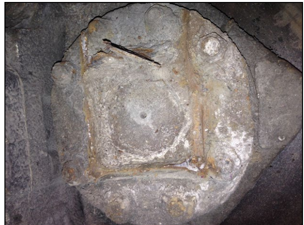
FIGURE 5: HEAVILY CORRODED COACH WITH BROKEN TAG AXLE. THIS IMAGE SHOWS THE SPINDLE MOUNTING PLATE SEPARATED FROM THE REST OF THE TAG AXLE
