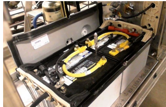
FIGURE 47: BATTERY BANK COVER REMOVED
