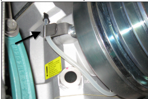
FIGURE 1: SHAFT SEAL OIL COLLECTION TUBE
