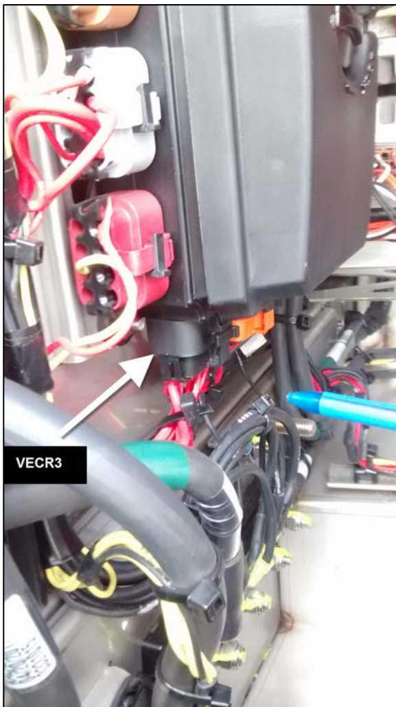
FIGURE 25: REAR JUNCTION BOX
