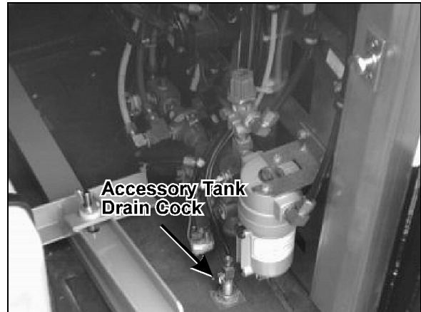
FRONT SERVICE COMPARTMENT
