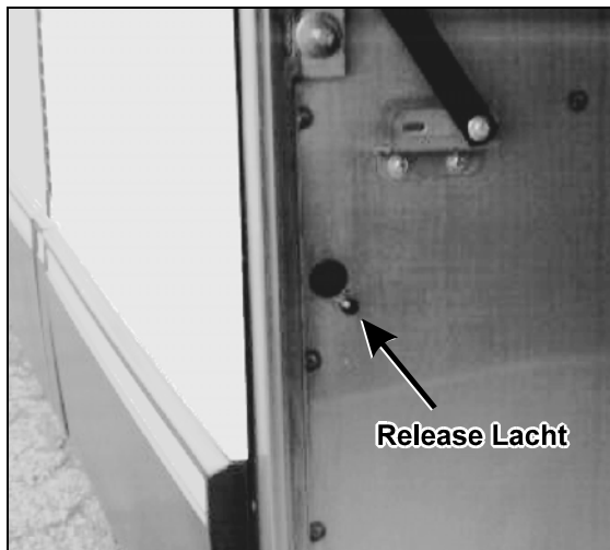
HVAC COMPARTMENT ACCESS
