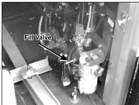
FILL VALVE IN FRONT SERVICE COMPARTMENT
