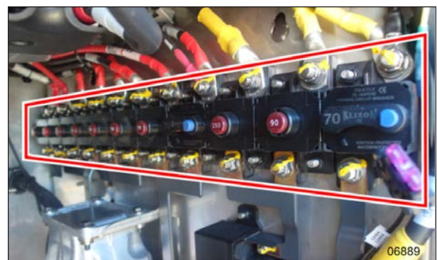
FIGURE 11: MAIN CIRCUIT BREAKERS IN MPC (TYPICAL)
