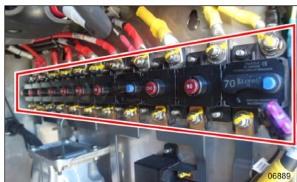
FIGURE 12: MAIN CIRCUIT BREAKERS IN MPC (TYPICAL)
