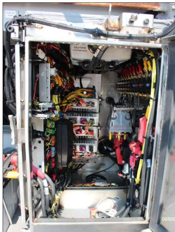
FIGURE 10: MAIN POWER COMPARTMENT (TYPICAL)
