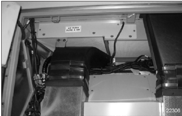
FIGURE 24: CABIN AREA AIR FILTER
