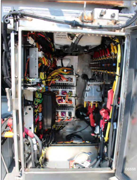
FIGURE 10: MAIN POWER COMPARTMENT (TYPICAL)
