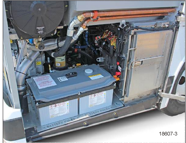
FIGURE 8: ENGINE COMPARTMENT R.H. SIDE
