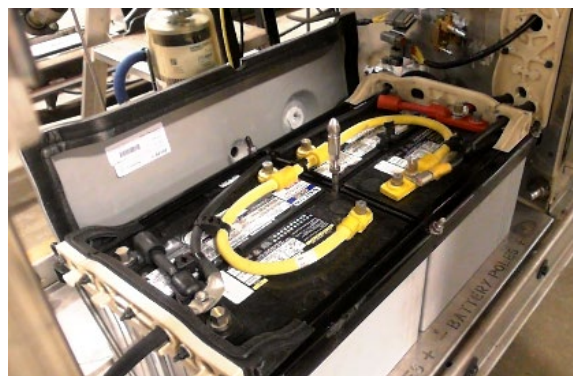
FIGURE 47: BATTERY BANK COVER REMOVED
