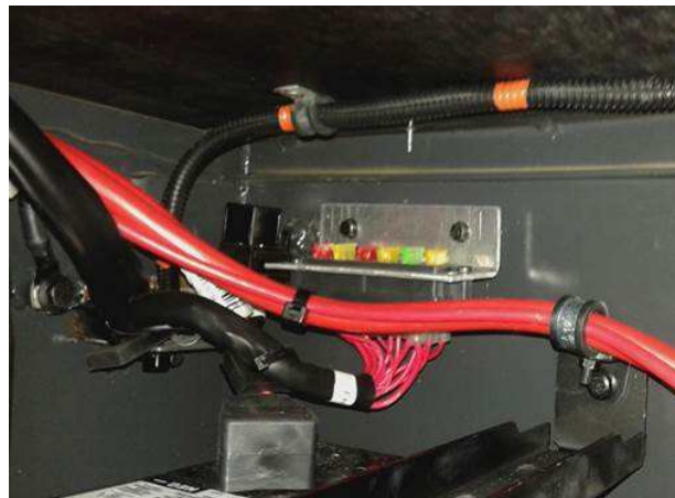
FIGURE 5 : For vehicles equipped with I-START dual battery system (from 3CET2V220G5177311 ), find K918 at the starter batteries compartment.
