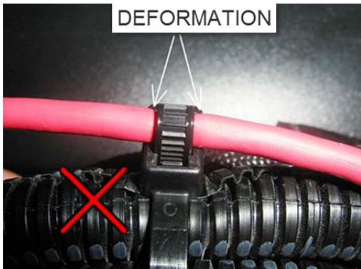
Cable tie tighten in excess on the LTD. Tighten cable tie on LTD by hand only. Tighten just enough to prevent LTD from slipping from one side to the other inside the cable tie loop
