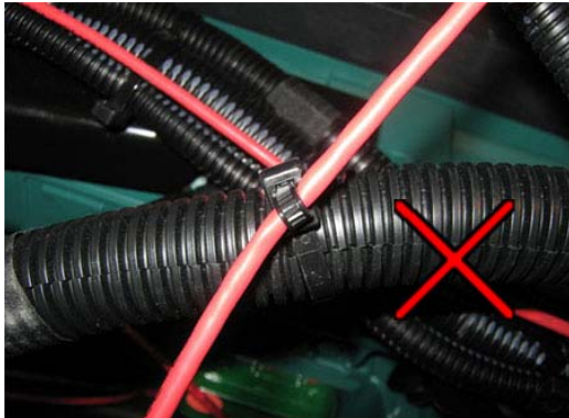
LTD extending slantingly from the cable tie
