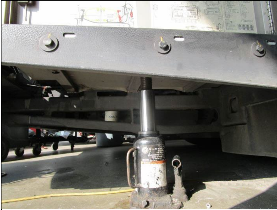
FIGURE 12: SUPPORTED BATTERY TRAY
