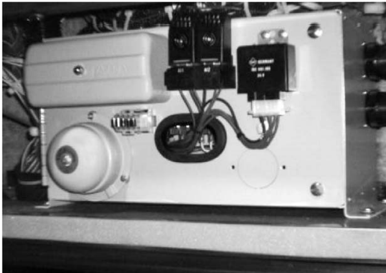
FIGURE 1: ALARM JUNCTION BOX
