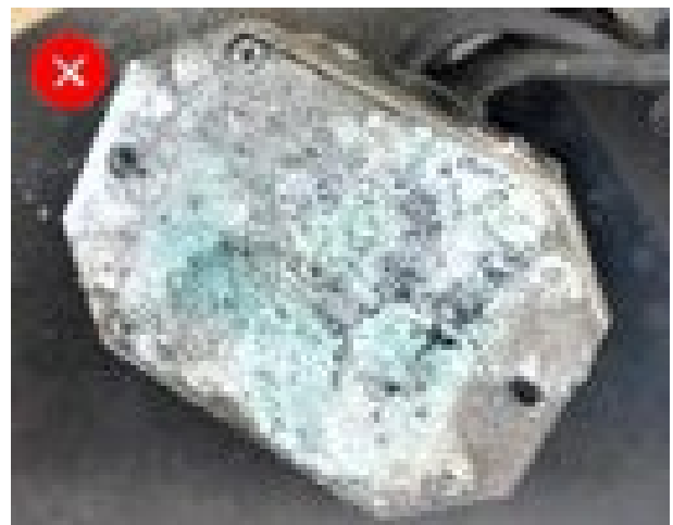
BACK SIDE COVERED BY CORROSION - REPLACE
