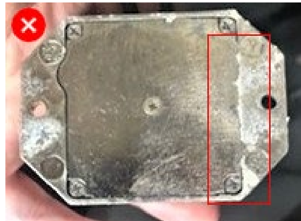
WHITE CORROSION AT ONE EDGE - REPLACE
