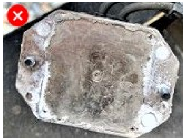
WHITE CORROSION ALL AROUND THE COVER - REPLACE
