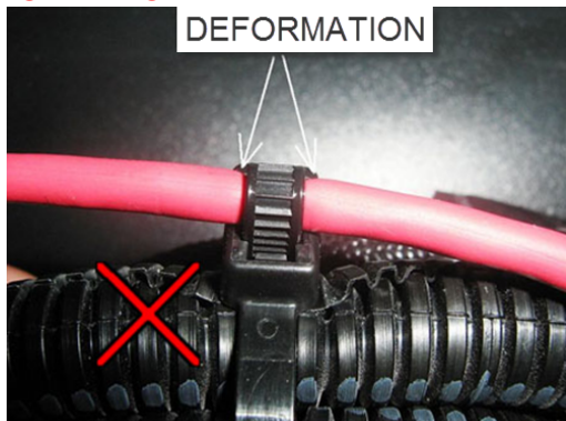
Cable tie tighten in excess on the LTD. Tighten cable tie on LTD by hand only. Tighten just enough to prevent LTD from slipping from once side to the other inside the cable tie loop
