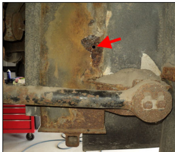
FIGURE 7: HOLE DRILLED IN STRUCTURAL MEMBER
