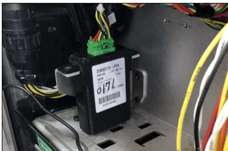
FIGURE 27: MODULE ELD INSTALLÉ
