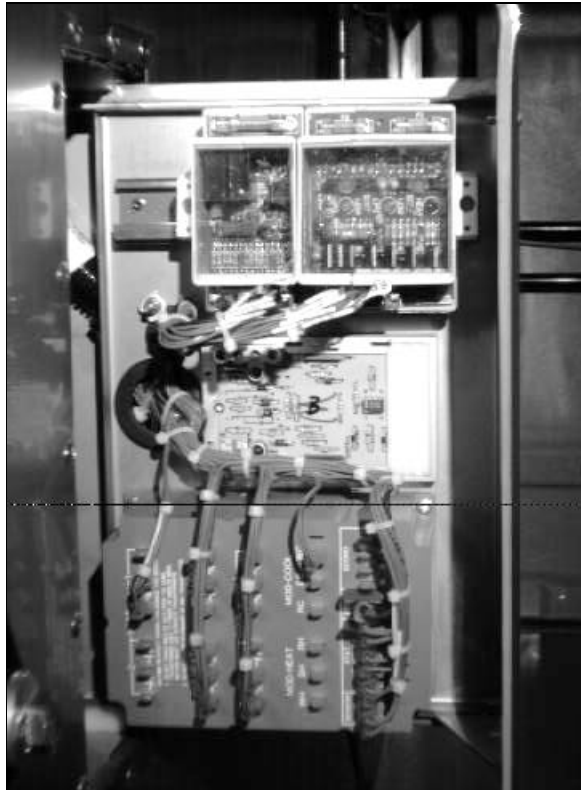
06062 FIGURE 5: A/C HEATING JUNCTION BOX SLIDING DRAWER
