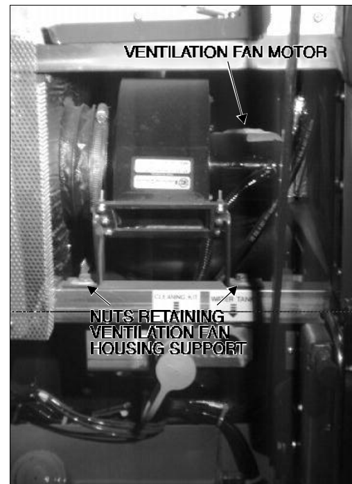
FIGURE 23: VENTILATION FAN MOTOR
