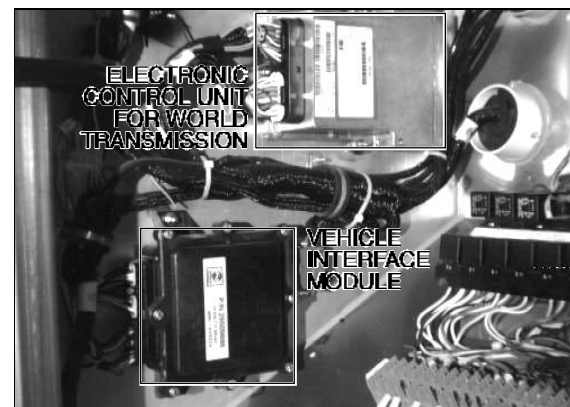
FIGURE 8: REAR ELECTRICAL COMPARTMENT 06055
