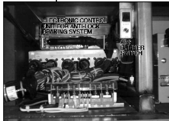
FIGURE 21: FRONT ELECTRIC COMPARTMENT 12051
