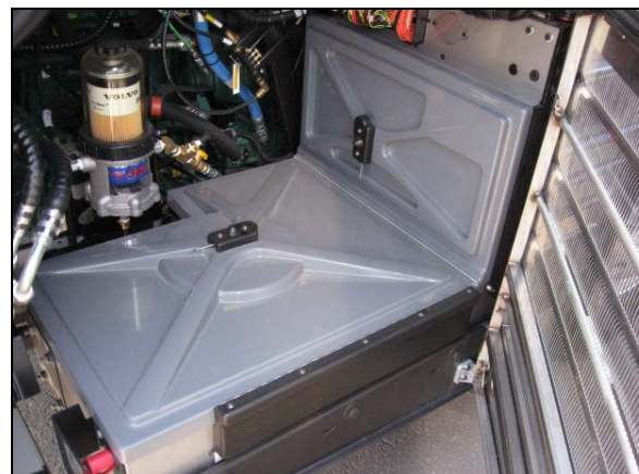
FIGURE 7: REAR ELECTRICAL PANEL, JUNCTION PANEL & BATTERY COMPARTMENT
