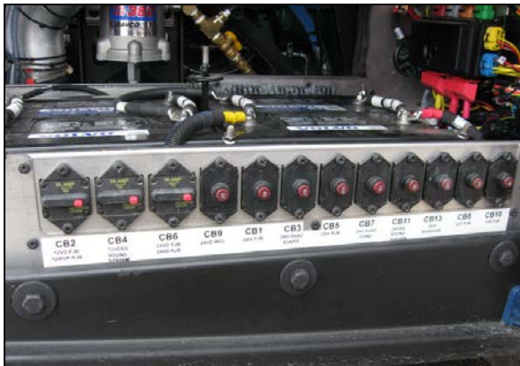
FIGURE 10: REAR ELECTRICAL JUNCTION PANEL
