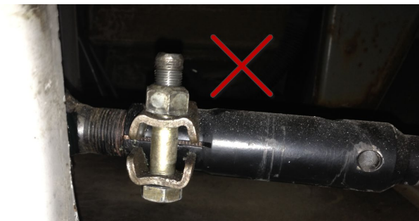
Clamp is bent. Replace clamp.
