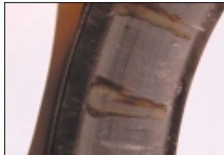
Cup shows considerable corrosion. This will develop in spalling.
