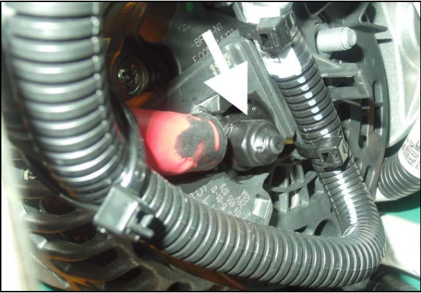
Figure 25: Lower alternator power cable lug protected with Color Guard rubber coating.
