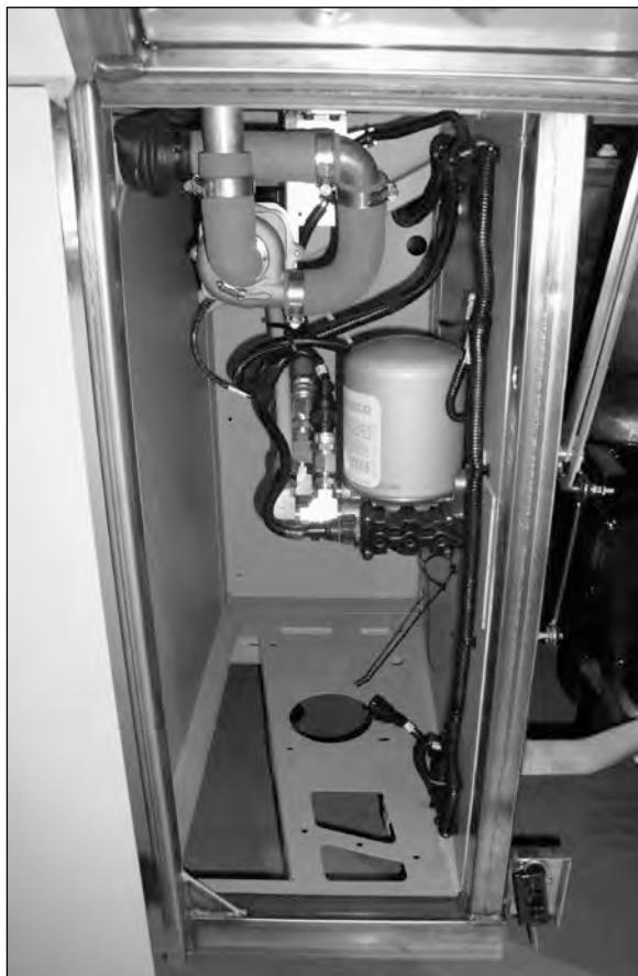
COOLANT HEATER COMPARTMENT
