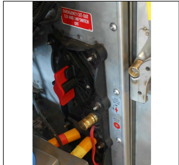
BATTERY MASTER SWITCH
