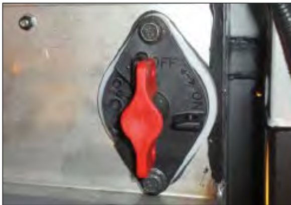
BATTERY MASTER SWITCH
