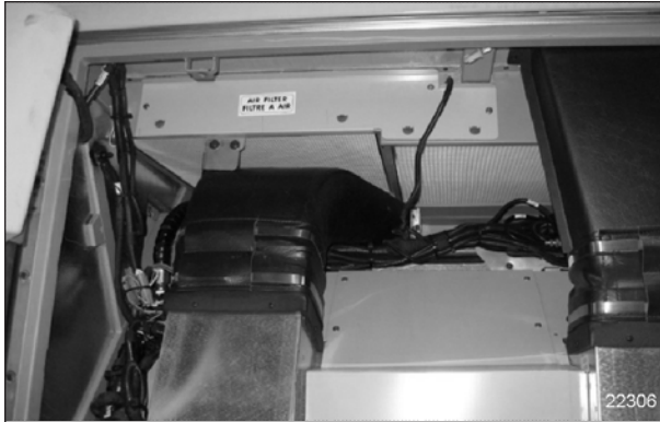
CABIN AREA AIR FILTER REMOVAL
