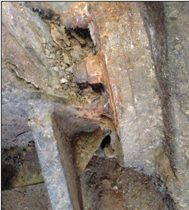
FIGURE 4: METAL FLAKING ON TAG AXLE - ACCUMULATED MATTER WILL RETAIN WATER THUS CREATING CONDITIONS PROMOTING ADDITIONAL CORROSION
