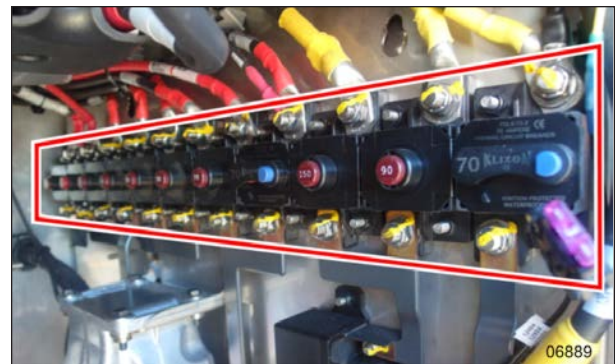
MAIN CIRCUIT BREAKERS IN MPC (TYPICAL)
