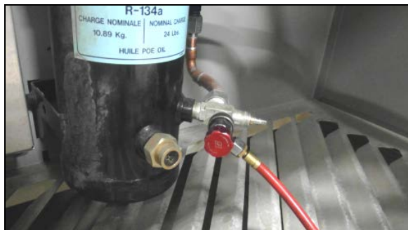
FIGURE 83: RECOVERY UNIT CONNECTED TO RECEIVER SERVICE PORT
