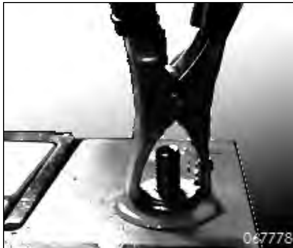
FIGURE 46 ALLIGATOR CLAMP POSITION- TYPICAL AGM BATTERY
