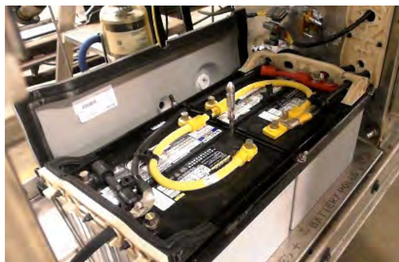
FIGURE 31: BATTERY BANK COVER REMOVED
