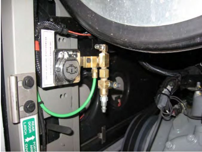
Figure 23: ENGINE COMPARTMENT EMERGENCY AIR-FILL VALVE
