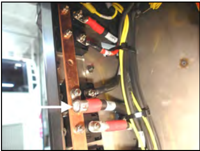
Figure 11: Power cable on main circuit breakers' bus bar.
