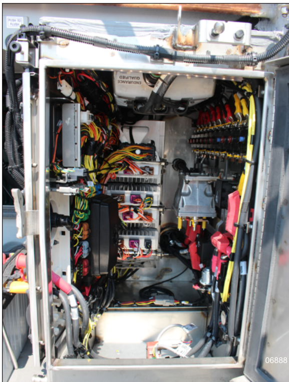
FIGURE 10: MAIN POWER COMPARTMENT (TYPICAL)
