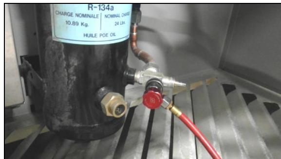
FIGURE 83: RECOVERY UNIT CONNECTED TO RECEIVER SERVICE PORT
