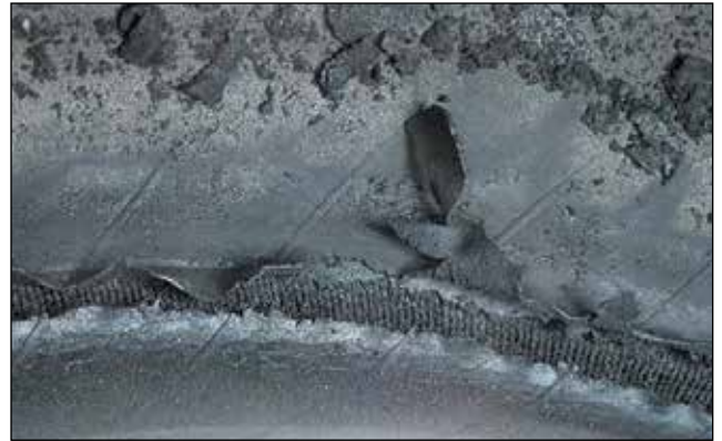
Inner Liner Damages
