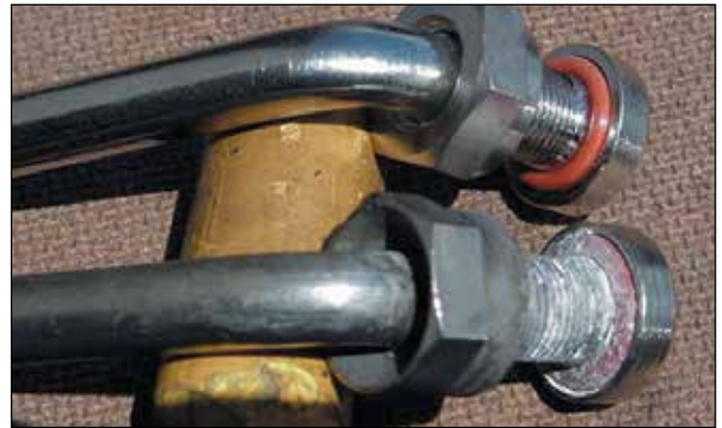
Note Corrosion On Bottom Valve
