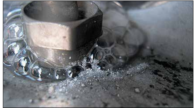
Corrosion Related Leak at the Base of the Wheel
