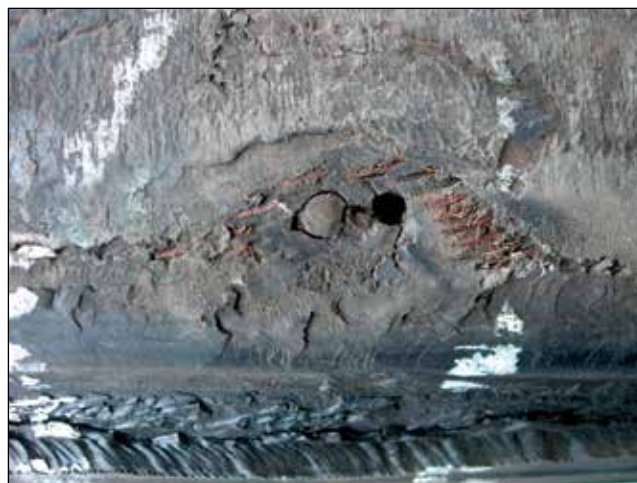
EFFECT: Missed Nail Hole CAUSE: Repaired from the Outside Resulting in Missed Damage
