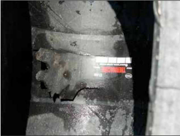
EFFECT: Improper Repair or Improper Repair Procedures CAUSE: Premature Failure of Repair
