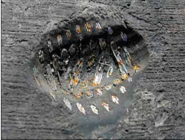
EFFECT: Exposed Steel Cord CAUSE: Detachment of Repair Product
