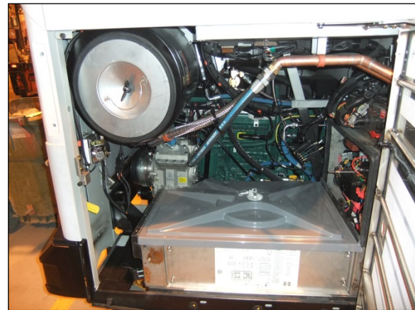
ENGINE COMPARTMENT R.H. SIDE
